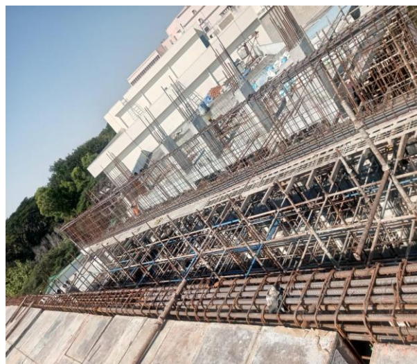
Fig 2. Congestion of Reinforcement in Roof Beam / Slab
