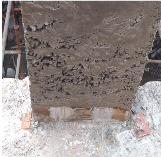
Fig 1. Typical illustration of Honeycombing in RCC members
