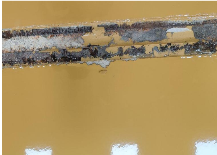
Fig 5. Error in laying ESD flooring at the steel and concrete interface
