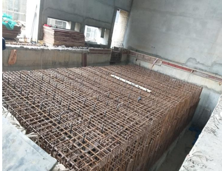
Fig 3. Reinforcement Congestion in Foundation Block
