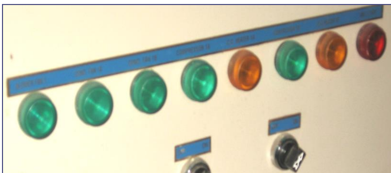
Figure 24: Pilot Lamp at Distribution Board
