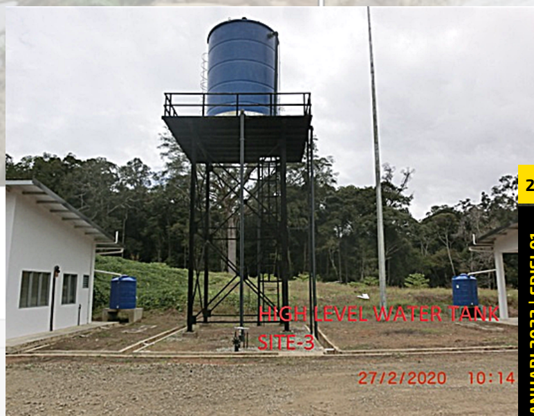
High Level Water Tank
