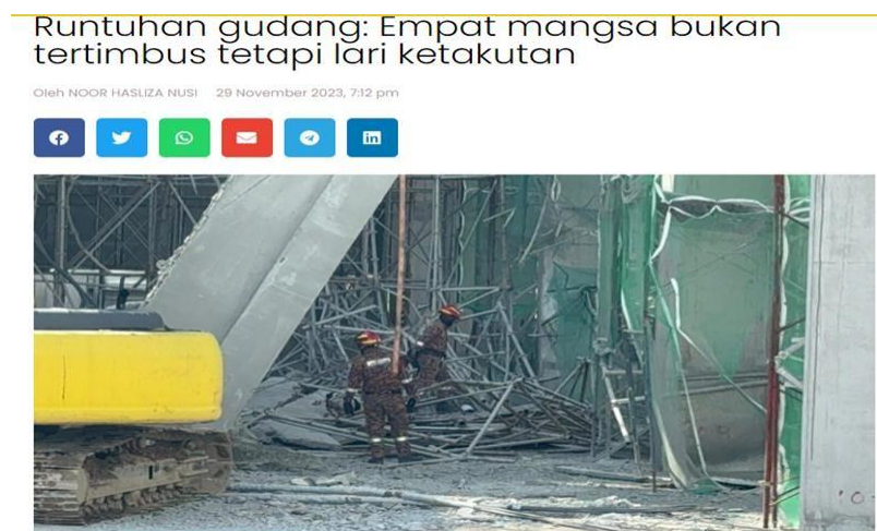
Figure 1.2: Accident at Construction Site
