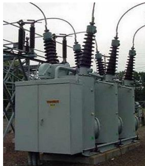
Figure 2.13 : Oil Circuit Breaker
