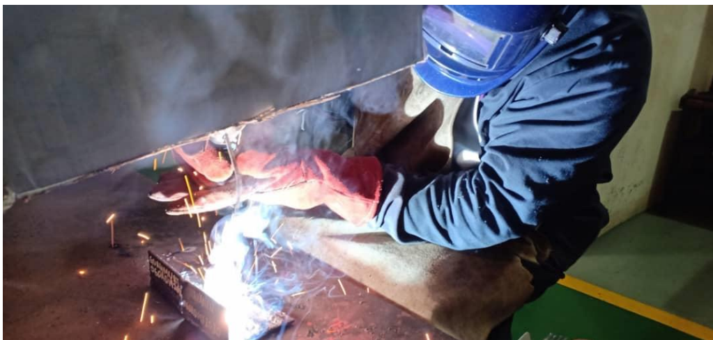
Figure 1: CO released during welding activity in workshop measured using CO meter AS8700A
