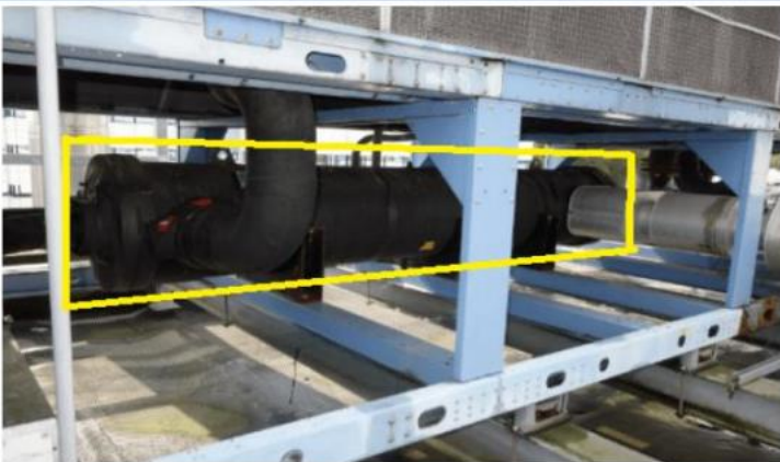
Evaporator on an air cooled chiller
