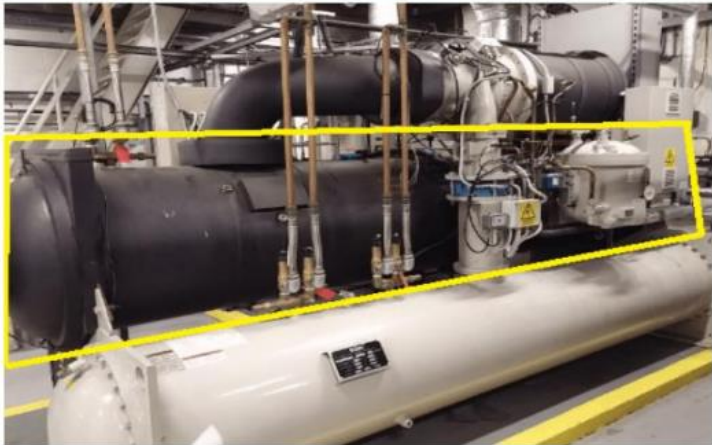
Evaporator on a water cooled chiller
