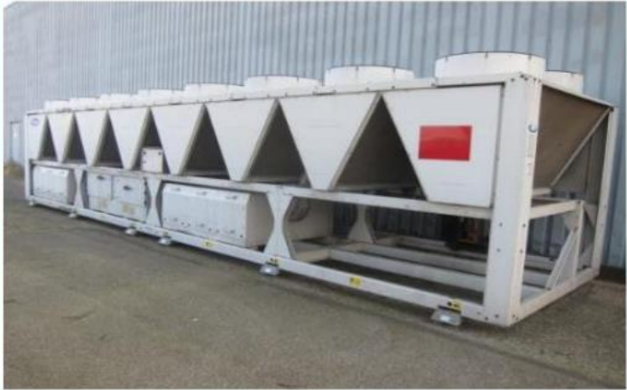
Air cooled chiller
