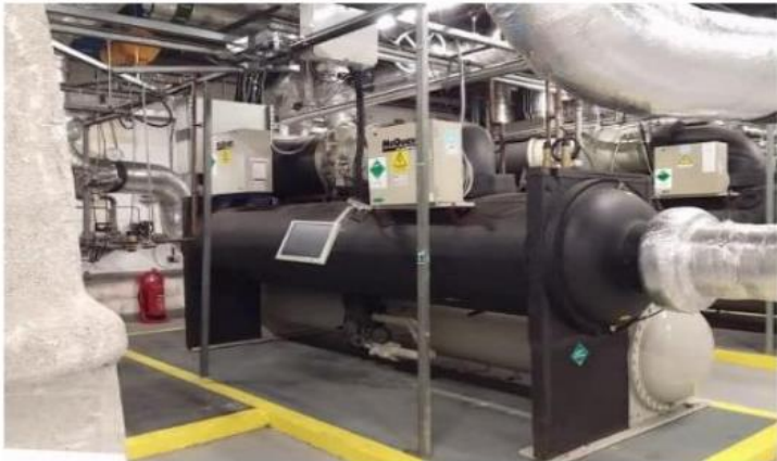
Water cooled chiller
