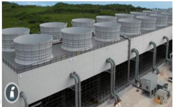
Mechanical Draft Cooling Towers
