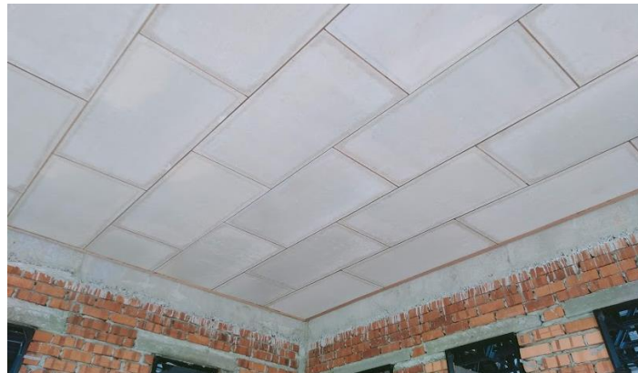
Rajah 88: Keadaan siling asbestos bahagian garaj kereta
