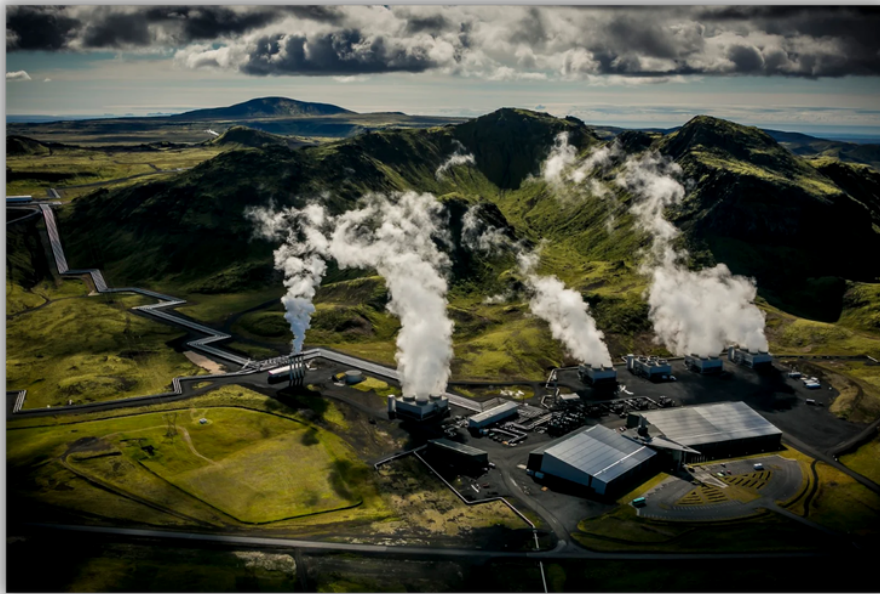
Rajah 1.8: Hellisheidi Geothermal Power Plant, South-West, Iceland
