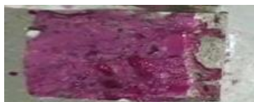
Figure 4.: Carbonation test sample of Beam 01
