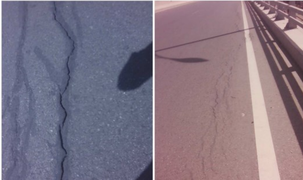
Figure 7: Cracks on Both Viaducts
