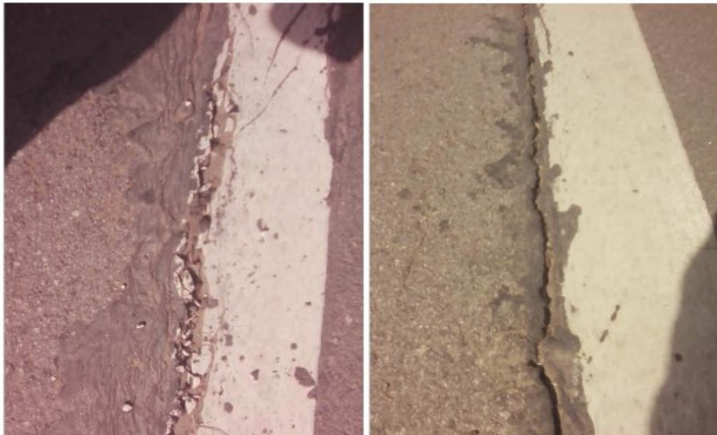
Figure 6: Edge Cracking during Viaduct Elevation.
